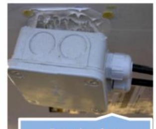
Junction box adhesion
