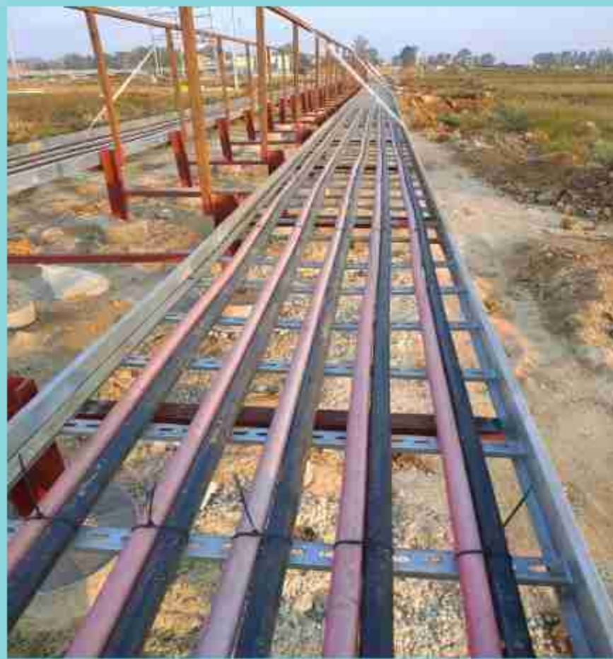
OVER CABLE TRAY
