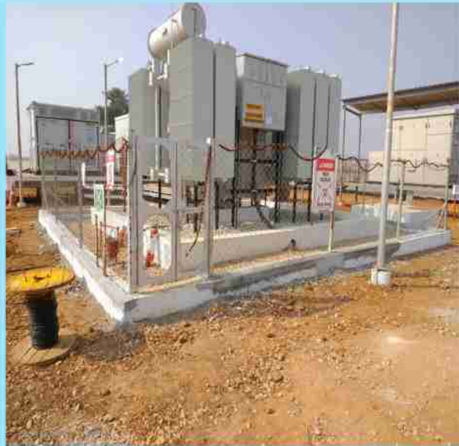
6.875 MVA Inverter Control Room
